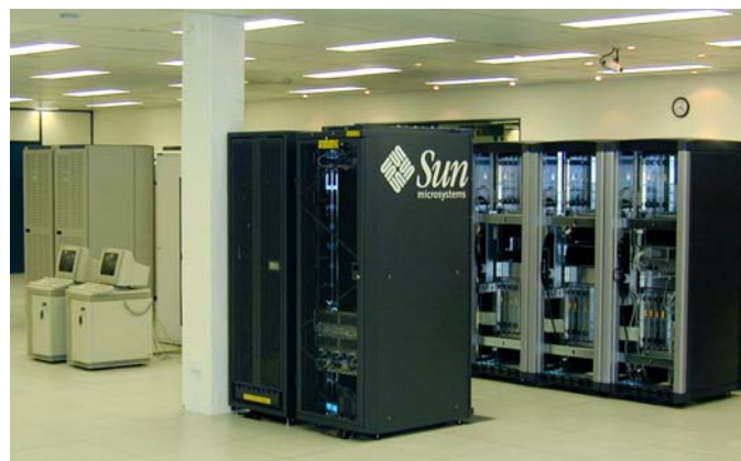
LPI Sun equipment located at ac3 .
